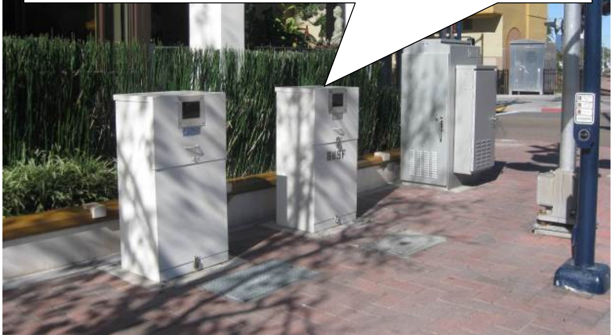
City Type 332 Traffic Signal Controller Cabinet with Battery Back-up Enclosure; Type III Service meter pedestal (2) – Different angle
